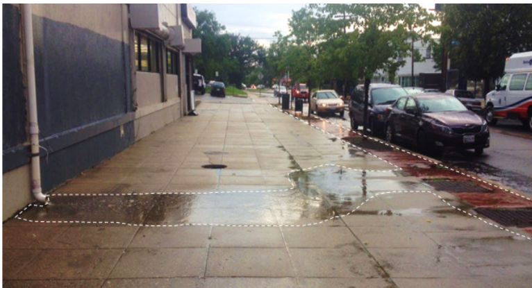
Before: Limited Infiltration on a Wide Sidewalk Resulting in Significant Runoff
