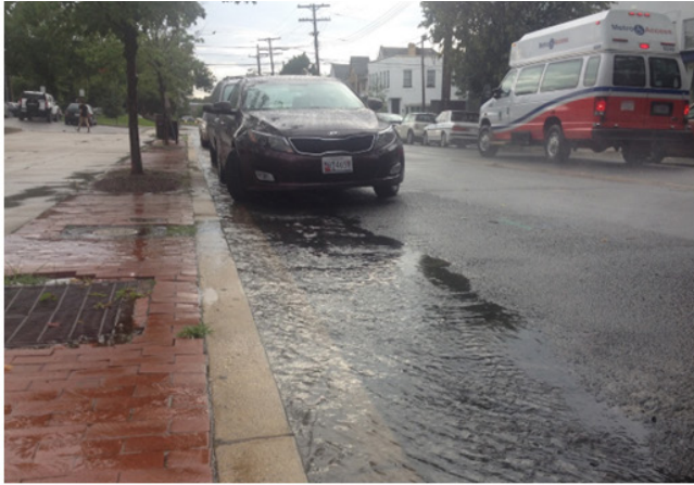
Before: All stormwater drains to gutter system, causing flooding and rapid runoff
